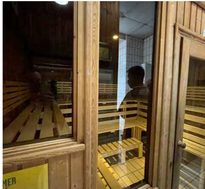
Sauna room, low quality fit-out materials, non original floor tiling.
