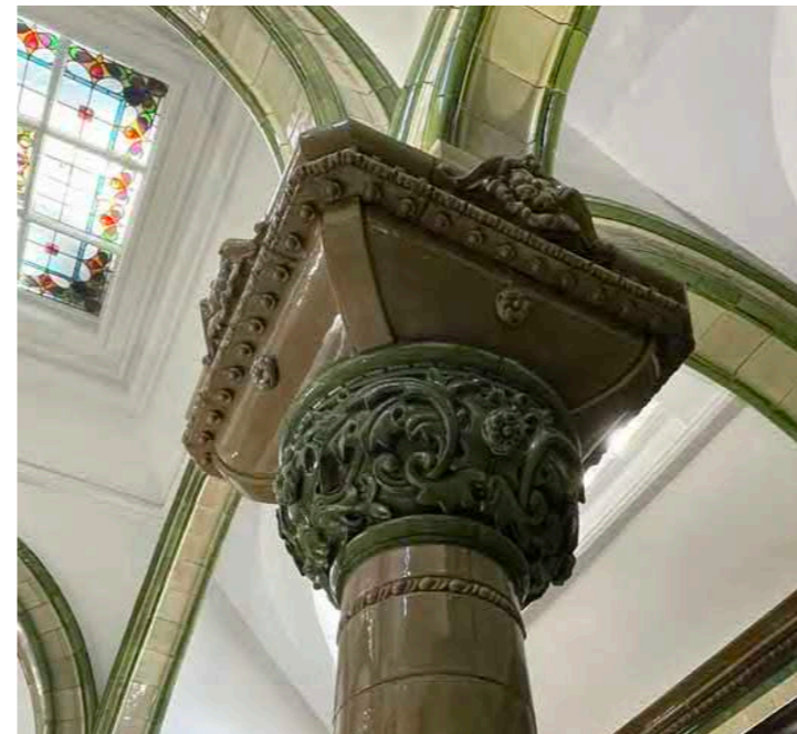
Decorative glazed tiling to column shaft, base and capital heads within the Turkish Baths.
