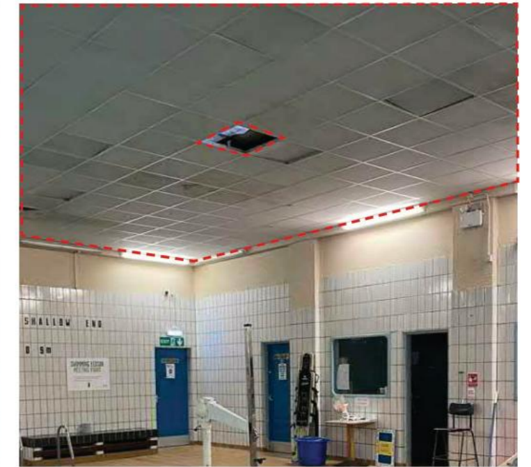
Suspended grid in-lay ceiling above the large/main pool ceiling tiles missing or damage/ lifting
