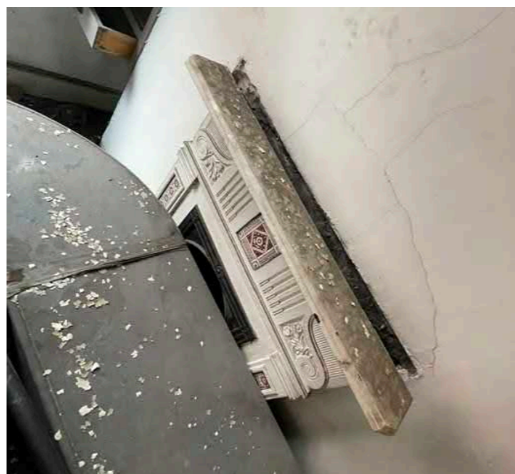
Duct work blocking original fireplace and hearth details.
