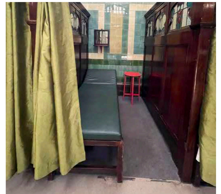
Existing changing booths with poor quality and degrading floor finishes.
