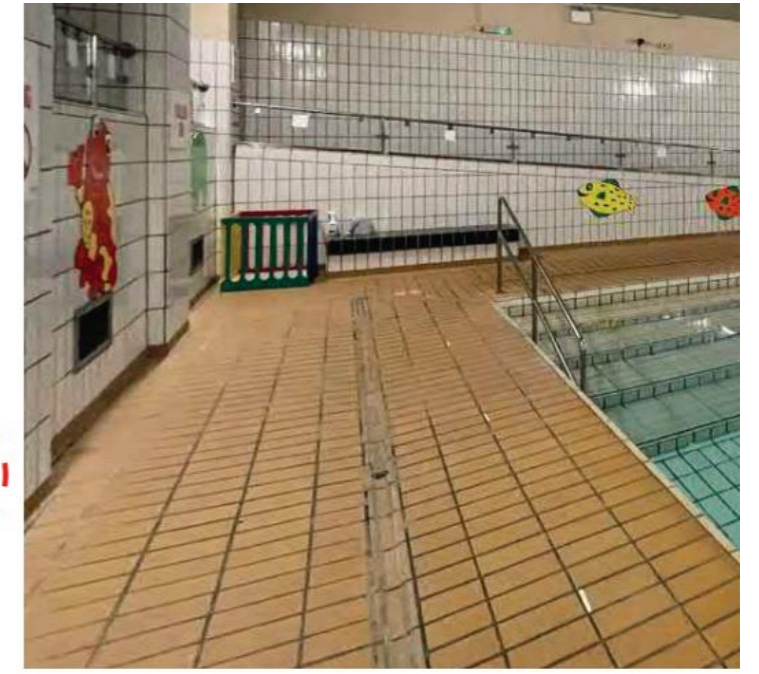
3. Draining floors to be made level and covered in suitable slip resistant fire retardant surface.
