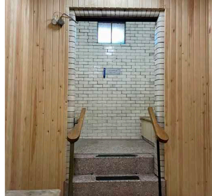
Areas of presumed original terrazzo flooring and glazed bricks, clad in poor quality timber coverings.
