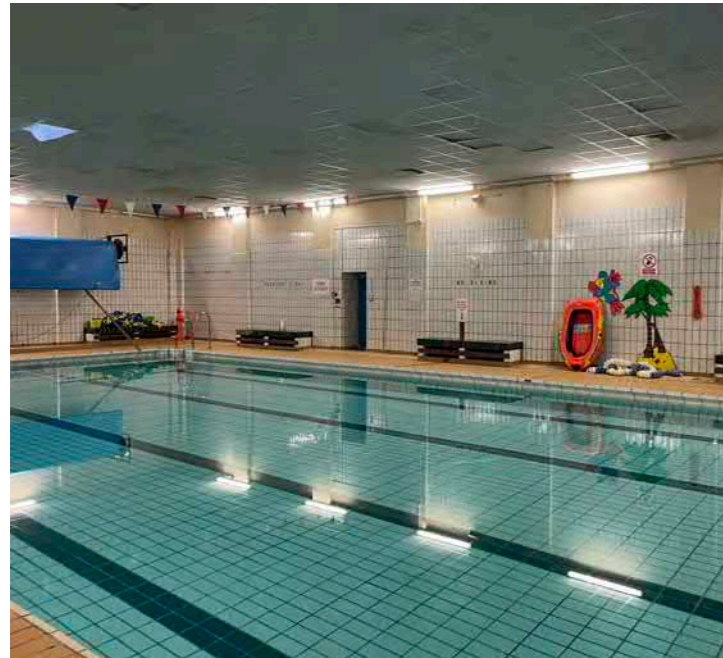
Large pool. Modern suspended ceiling, no evidence of visible historic finishes (ie. glazed brickwork, pool tiling).
