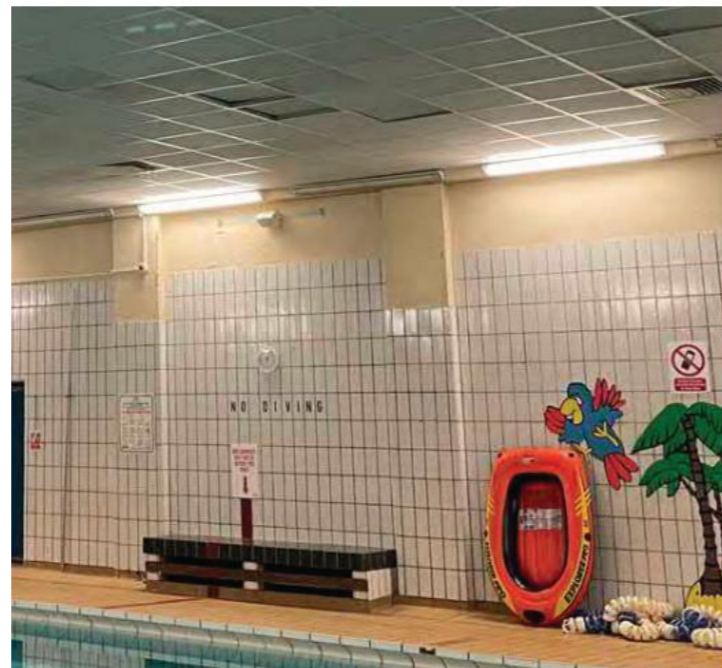
4. Wall hung lighting to be replaced.
