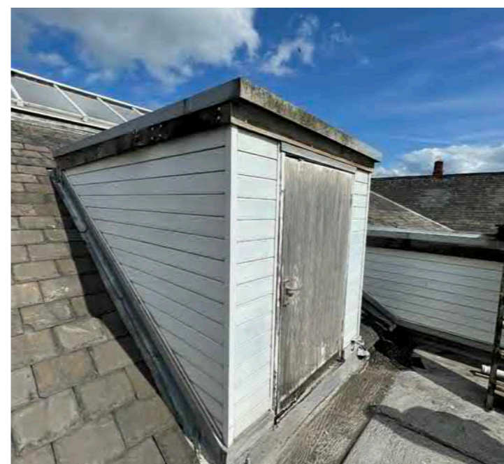
Poor quality roovescape additions, access hatches etc.
