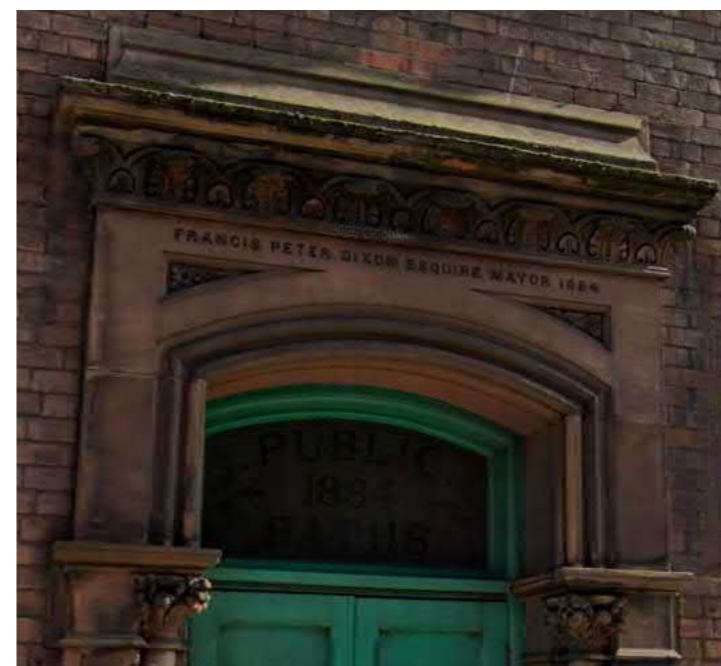
Masonry mouldings around the original entrance door. Noting building opening date of 1884 by the elected Mayor.
