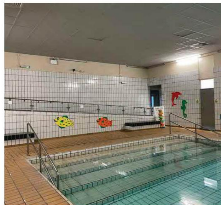
Suspended grid in-lay ceiling above the small (10m) pool showing signs of wear and deterioration
