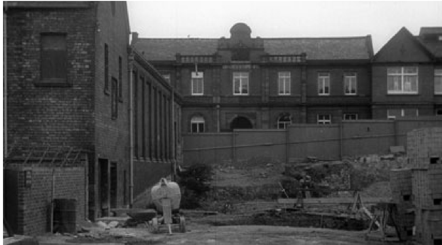
Figure 7: West elevation visible and foundations of the new Carlisle public baths, c.1974. Source: Cumbria Image Bank. ref: ct09040
