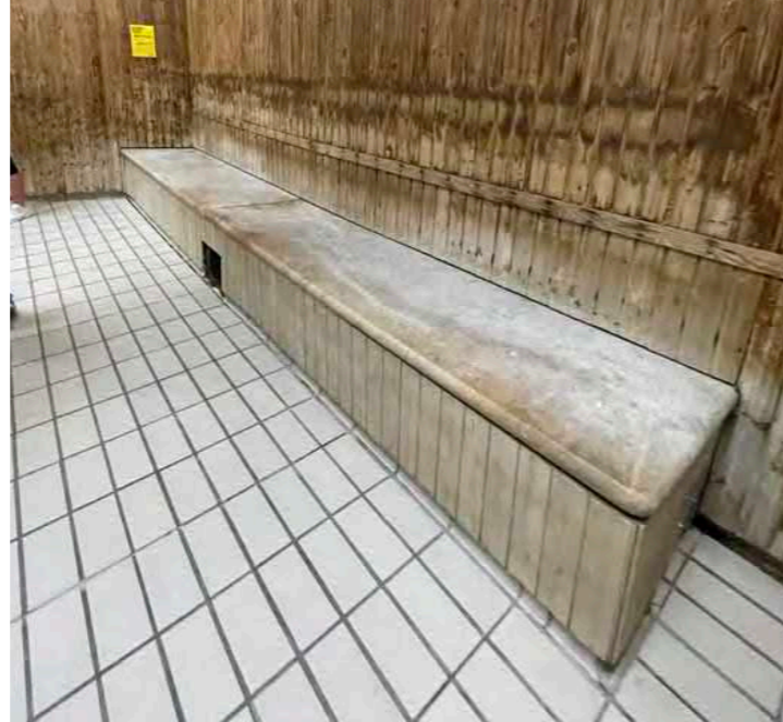
Marble topped sauna bench. Low quality and degrading wall linings and floor tiling.
