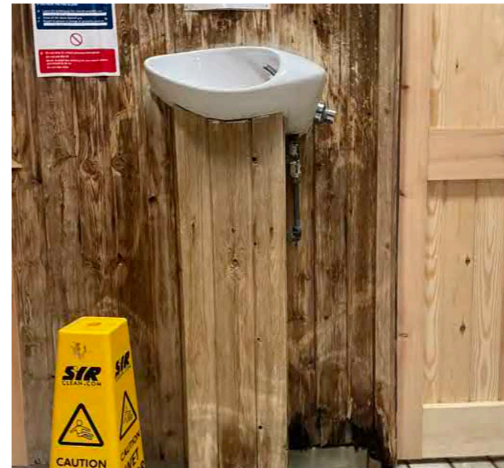
Sauna room, low quality fit-out materials showing signs of age and decay.
