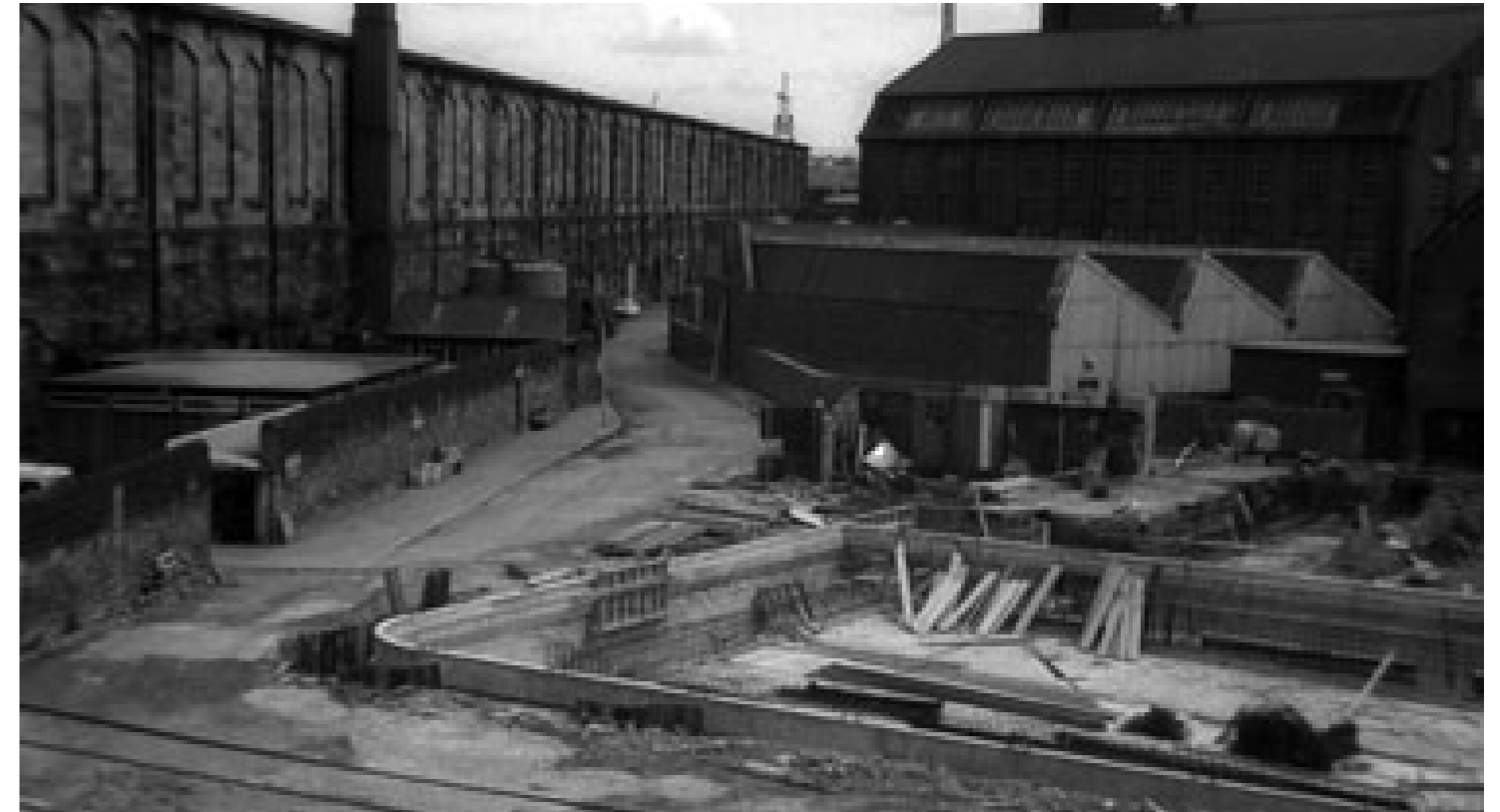
Figure 8: Foundations of the new Carlisle public baths, c.1974. Source: Cumbria Image Bank. ref: ct08301
