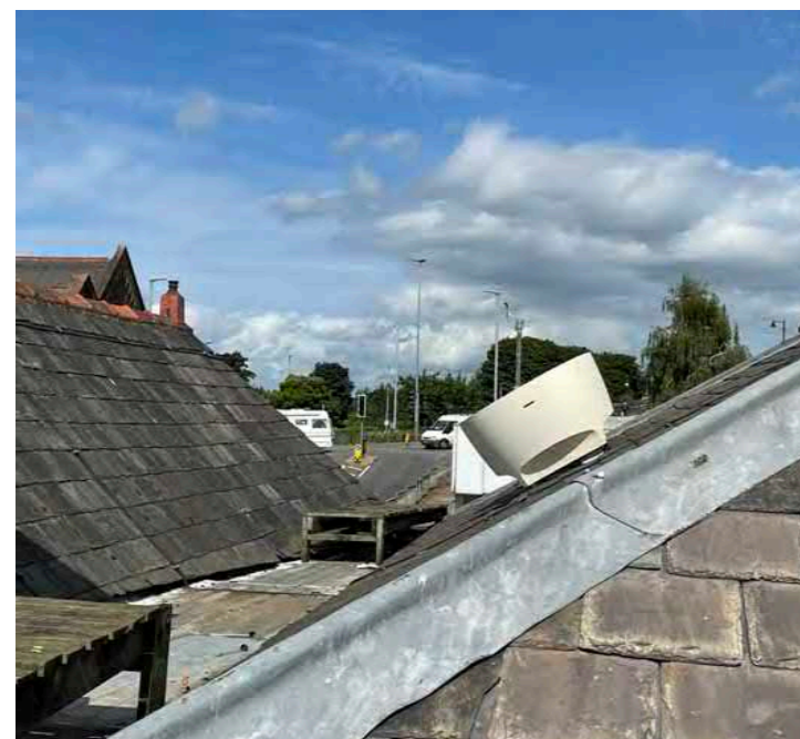
Poor quality roofscape additions, access gantries, security lighting.
