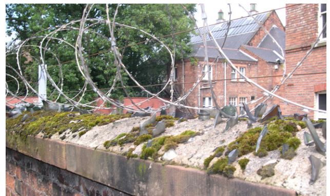
Fig 47. Inappropriate, crude security measures, City Centre.
