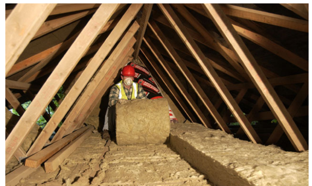
Fig 94. High levels of insulation is one of the key components of a sustainable building. 270mm of insulation is currently recommended. Energy Saving Trust
